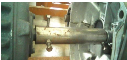
Fig.4: shaft coupled to motor and Gearbox
